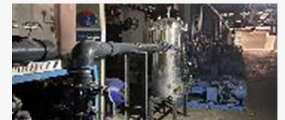
Xuzhou Xinyu Concentrated Water Recycling Unit
